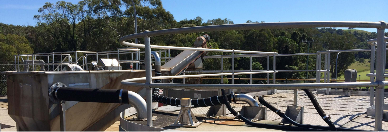
Wardell Wastewater Treatment Plant
