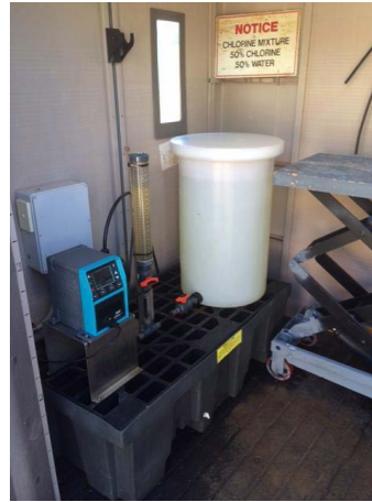
Chlorine is added to the water to fight any bacteria it may come into contact with before re-use.
