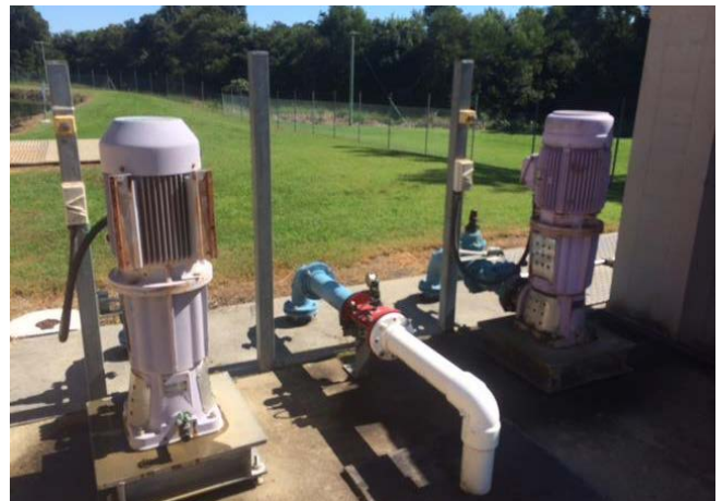
Pumps then send the recycled water to a reservoir where it is gravity fed to the following on-farm storages for irrigation purposes:
